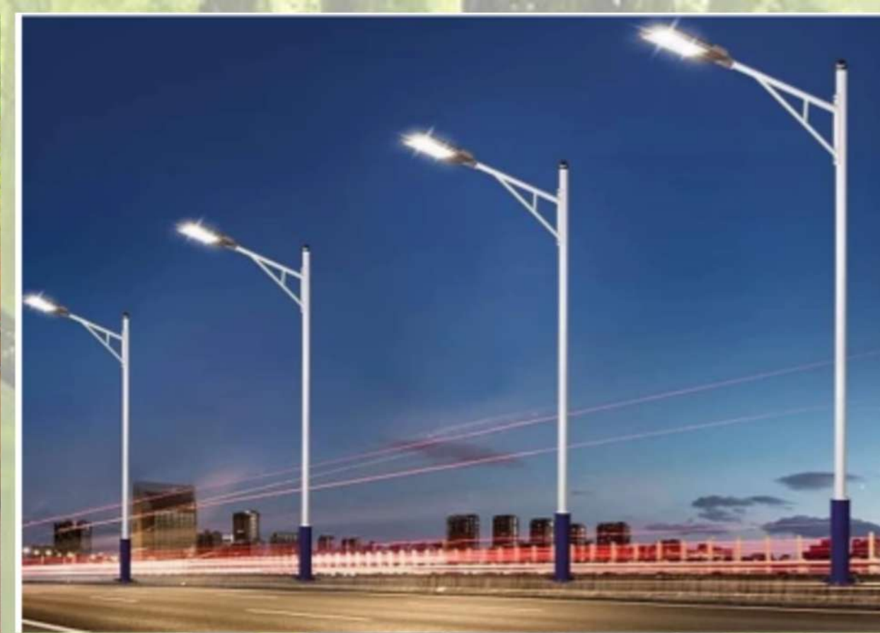
Roads and LED street lights
